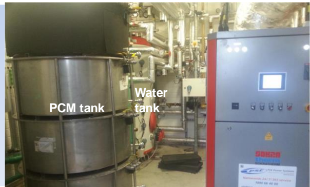
Heat Storage and CHP in the NIMBUS building, CIT
