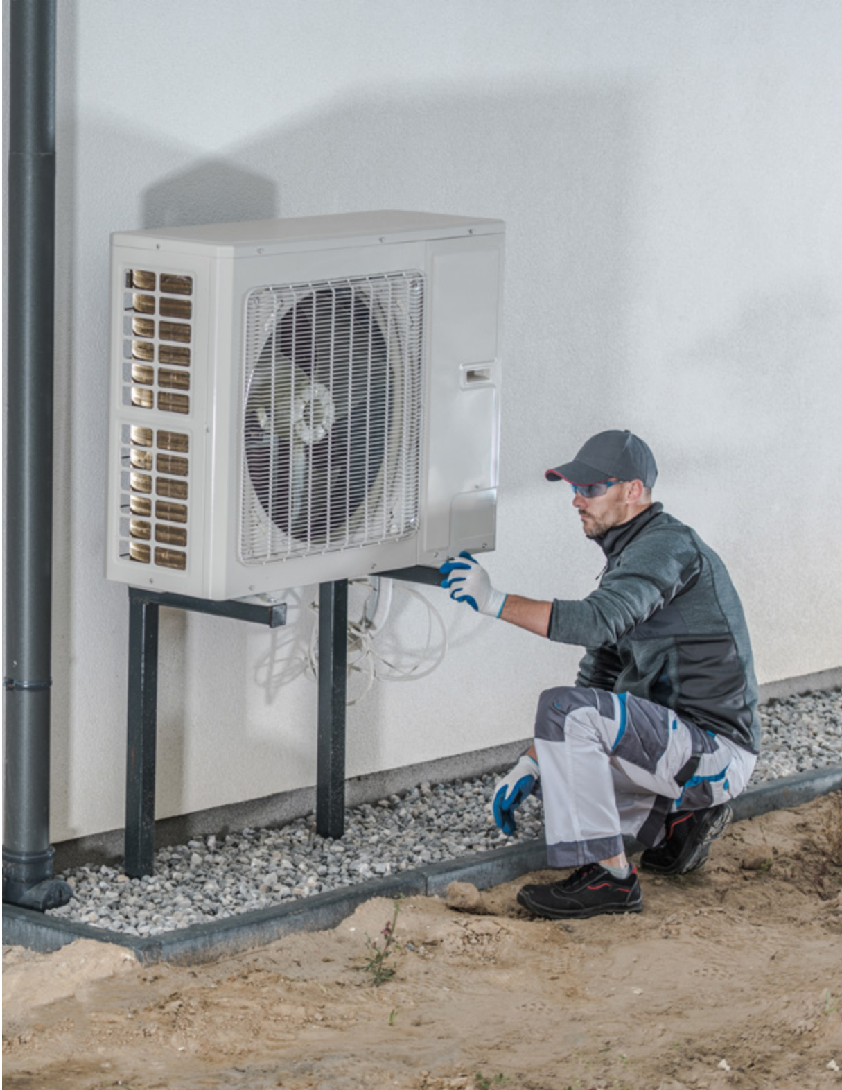
Figure 9: Outdoor heat pump unit
